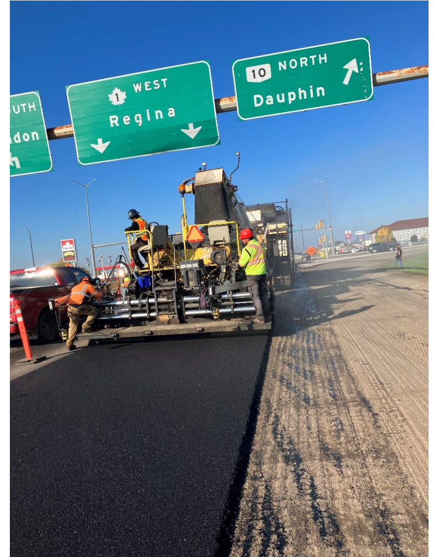
PTH 1: 0.3km W of W Jct PTH 10—0.3km E of E Jct PTH 10 Bituminous Rehabilitation
